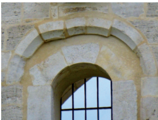
Figure 3. Dropped and repaired key stones in the window of the main apse of the Pujada de Santa María Church (Besalú).
